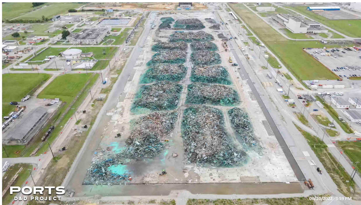
Figure 3.2. Demolition of the X-326 Process Building in June 2022 (looking north to south)
