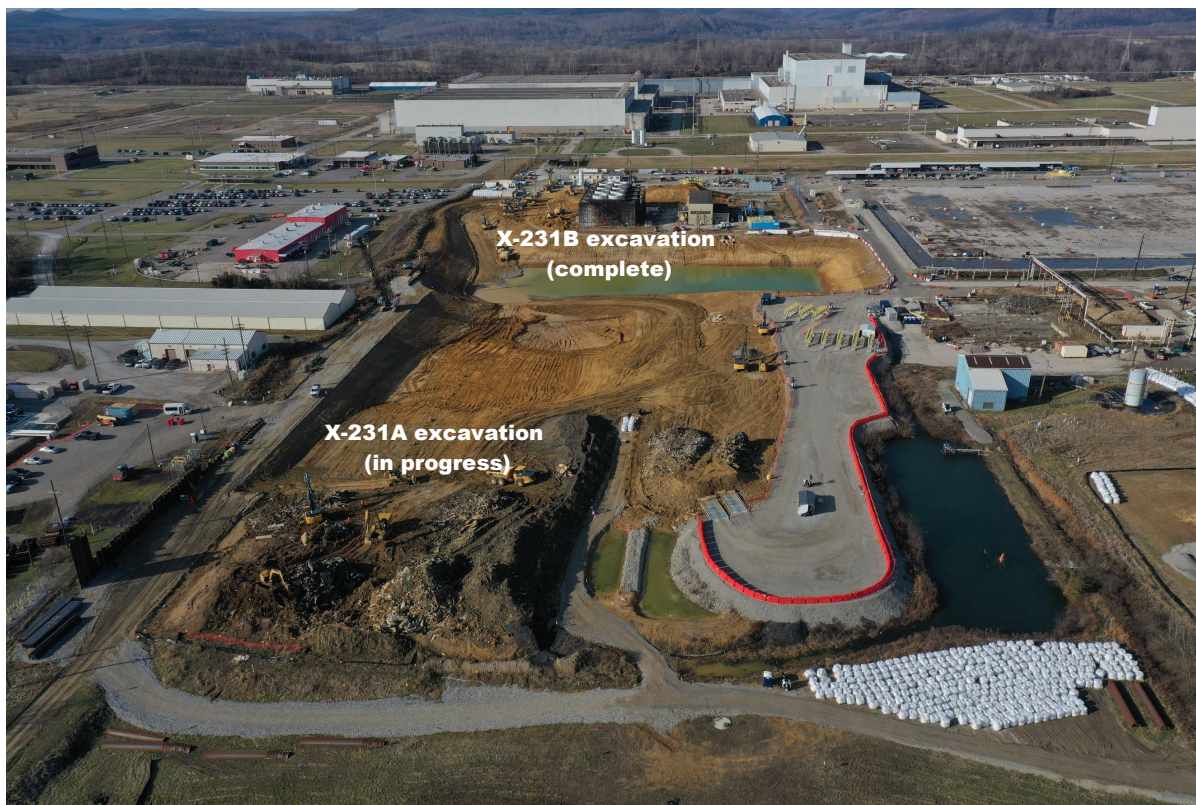
Figure 3.4. Excavation area at the Quadrant I Groundwater Investigative (5-Unit) Area in December 2022 (looking east to west)
