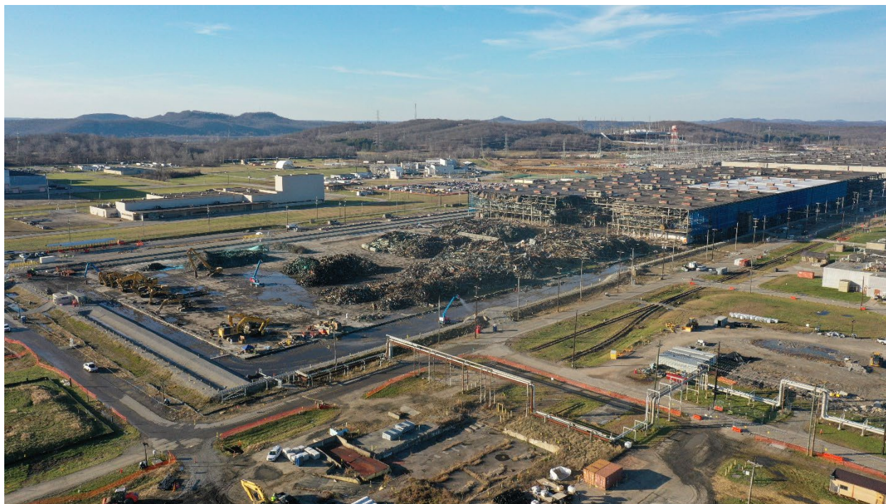
Figure 3.1. Extent of demolition of the X-326 Process Building in December 2021 (looking northwest)
